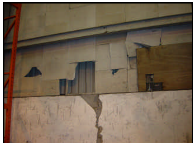
Photo showing broken cladding of "Asbestos Containing Material"
